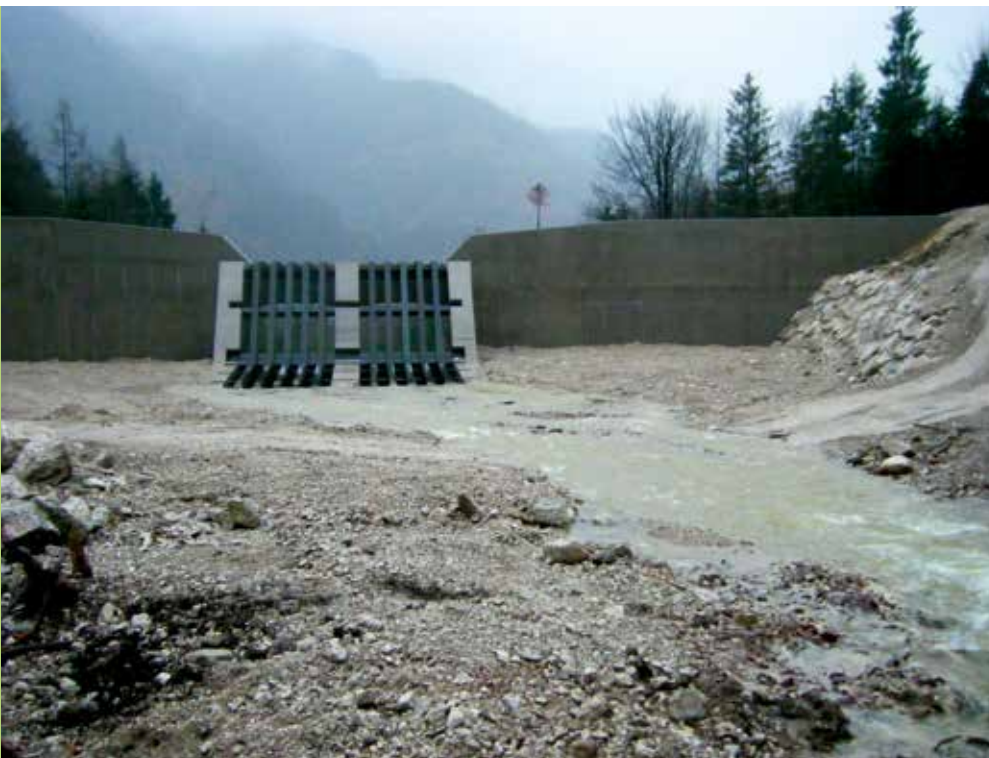
Fig. 9: Upstream view of the filtering structure including sorting rake
