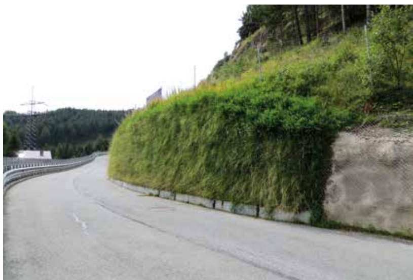
Fig. 1: Shotcrete wall including greening systems without vegetation (above) and shotcrete wall including greening systems with vegetation (below)
